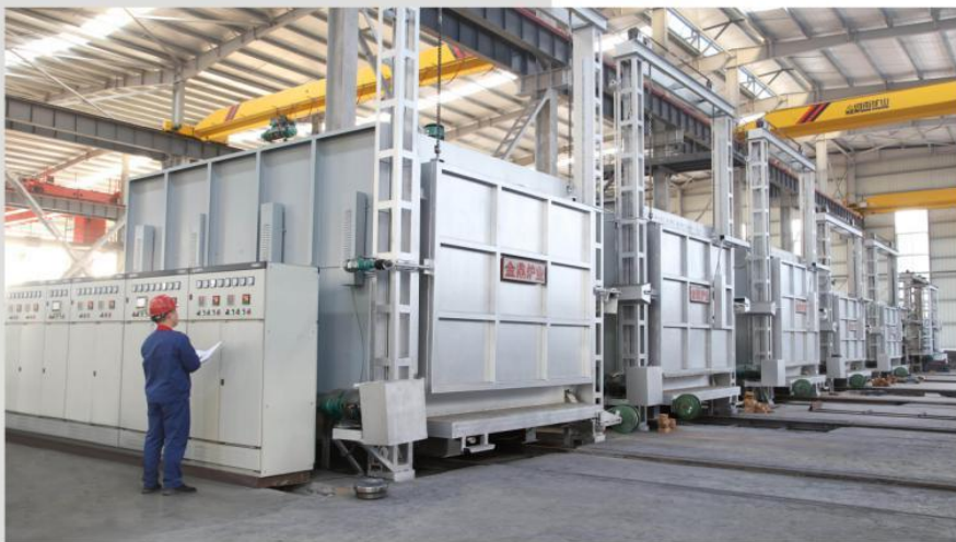
▲ 退火炉（热处理设备） Annealing furnace (heat treatment equipment)
